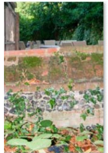
Churchyard wall poor repairs 3
